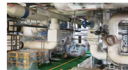
Waste Heat Station Colored Point Clouds
